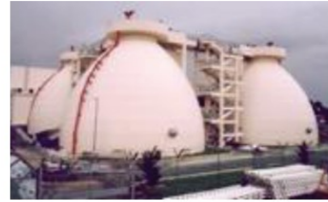
Kim Chuan Sewerage Treatment Plant, Singapore
