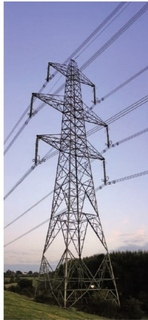
Electricity Power Line
