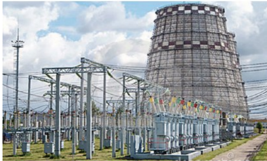
Electricity Power Plant Cooling Tower
