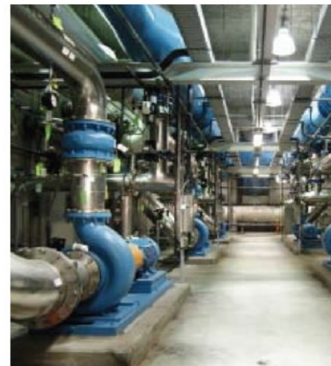
Sengkang West Sewage Lift Station, Singapore
